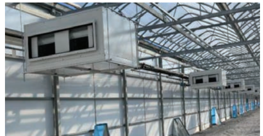
Air handling units at Daybreak Cannabis in St. Louis, MO.
