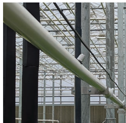
Co2 is safely distributed through nozzles.
