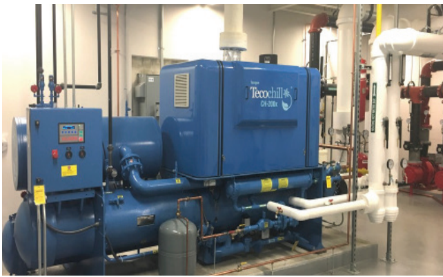
Tecogen's TecoChill line of natural gas engine driven chillers with free engine waste heat recovery is a form of mechanical CHP. Pictured above is a 200-ton Tecochill STx series chiller providing chilled glycol and hot water for dehumidification.
