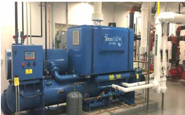
Tecogen's TecoChill line of natural gas engine driven chillers with free engine waste heat recovery is a form of mechanical CHP. Pictured above is a 200-ton Tecochill STx series chiller providing chilled glycol and hot water for dehumidification.
